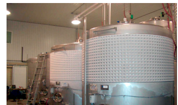
WINERY CHILLER SYSTEMS
